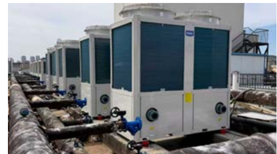
Solar and Air-Source Energy System
