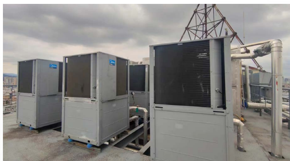
Modified Air-Source Energy System
